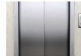
LIFT Kone / Schindler / Johnson / Otis or equivalent
